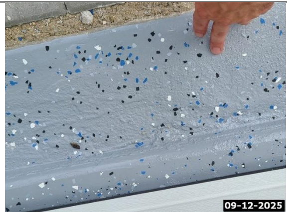
Debris Under Coating (Uneven)
