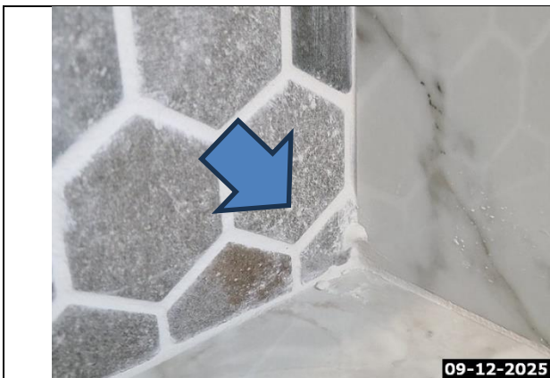
Grout on Tile at Shower
