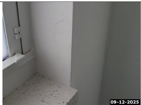
Poor Wall Texture Master Bathroom Window
