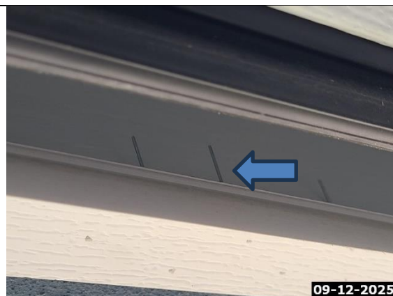
Nails Improperly Installed at Trim Around Garage Door Opening
