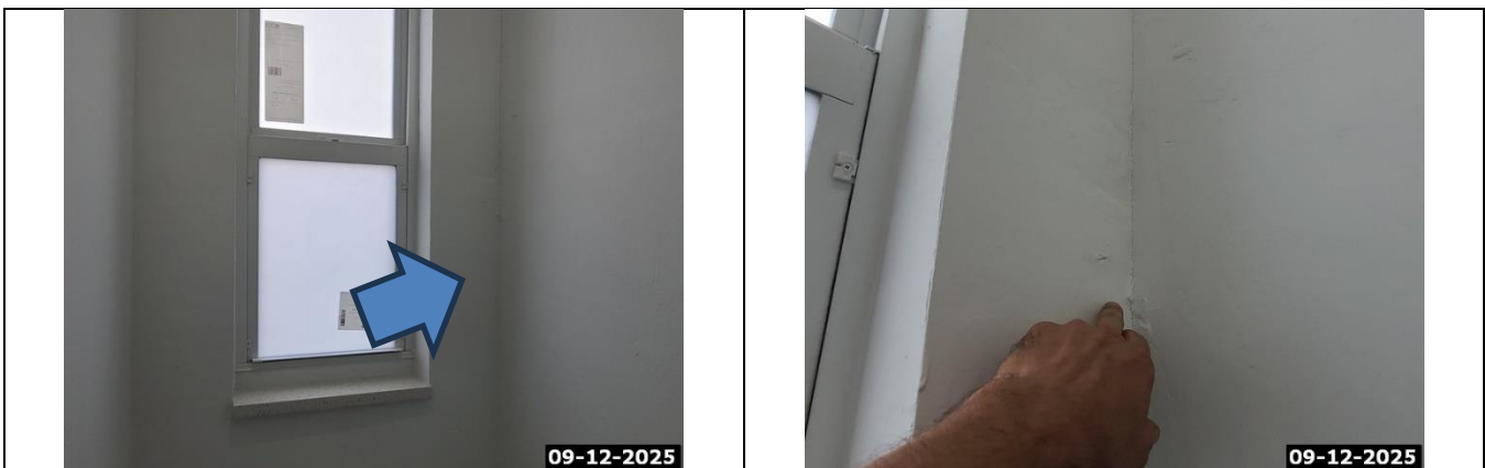
Thick, Poorly Installed Wall Texture
