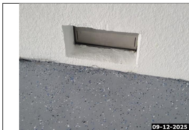
Openings for Garage Wall Vents are Not Perfectly Square and Have Poorly Installed Paint
