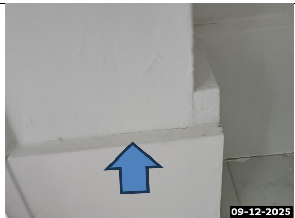
Cracking at Paint
