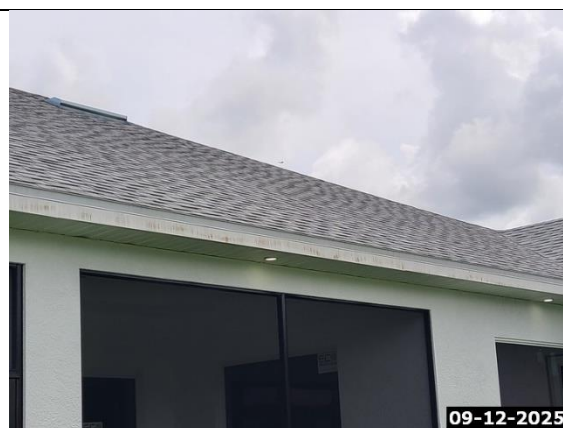
Staining at Fascias
