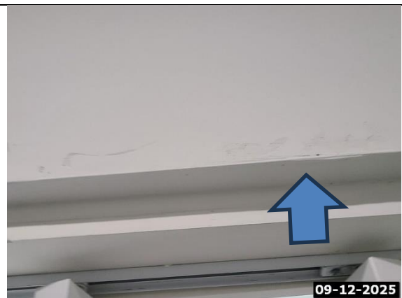
Poor Wall Texture
