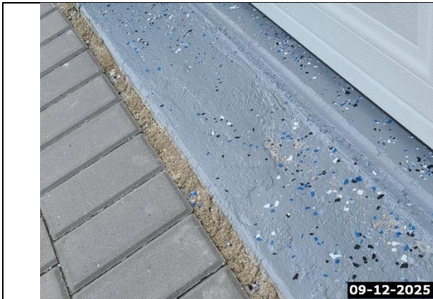
Debris Under Coating (Uneven)
