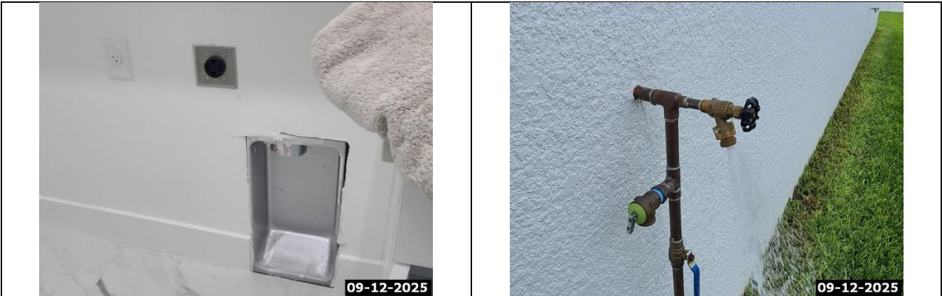
Plumbing System Images Plumbing System Images
