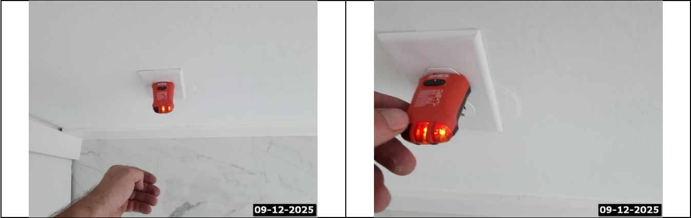
Wall Damage Near Outlet
