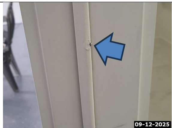
Damaged Weather Seal at Door
