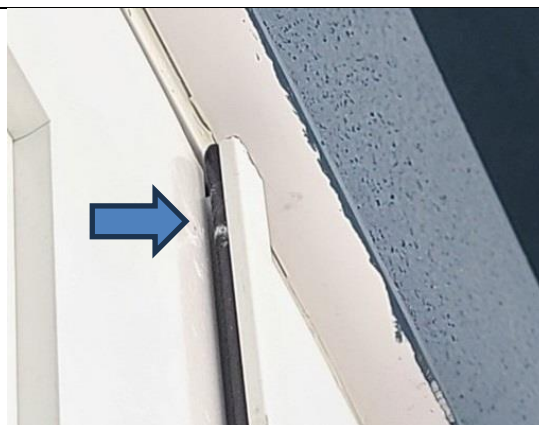
Gap at Door Astragal
