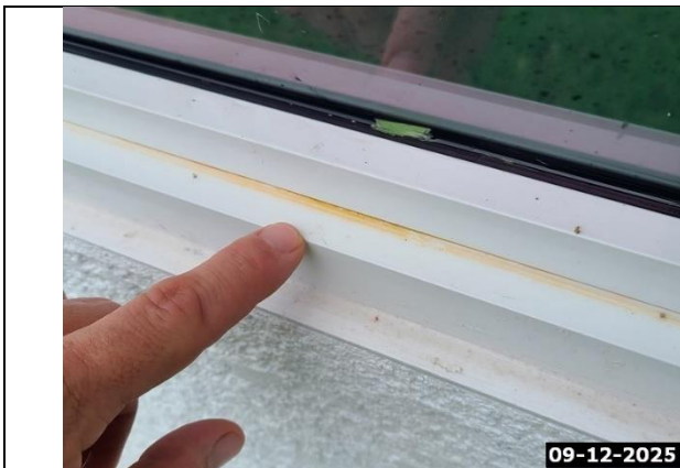
Staining at Seam Under Window Trim
