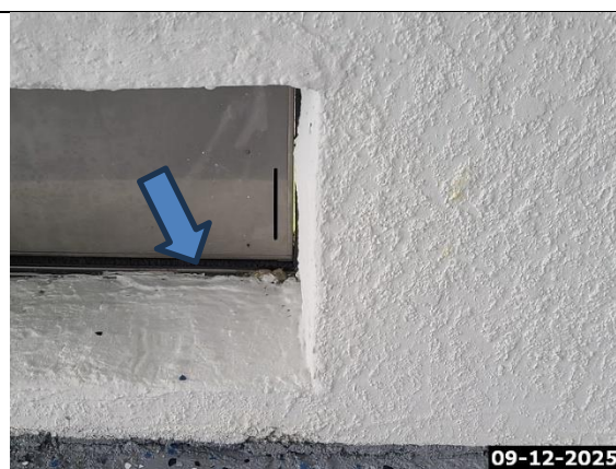
Openings for Garage Wall Vents are Not Perfectly Square and Have Poorly Installed Paint
