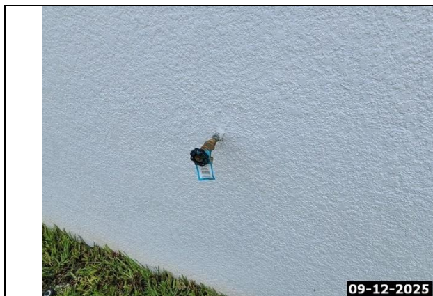
Cracking at Sealant
