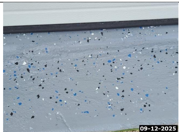
Debris Under Coating (Uneven)
