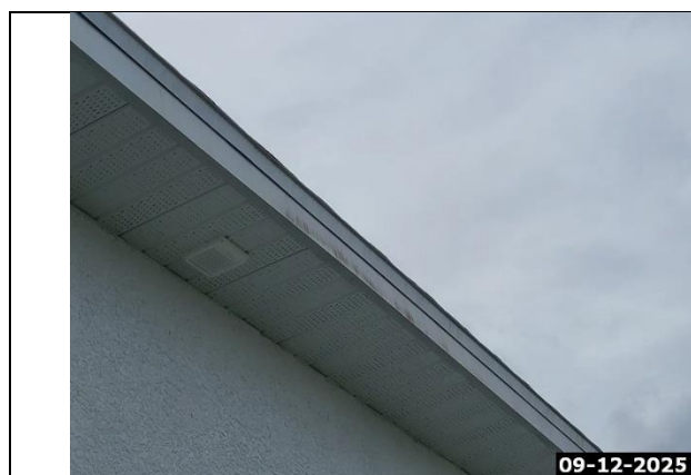
No Gapping at Areas of Drip Edge
