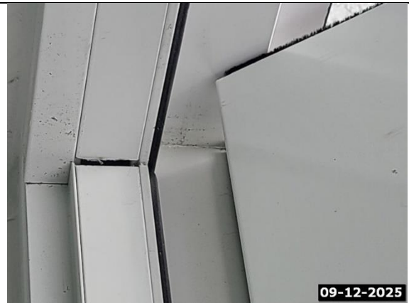
Gap at Door Frame
