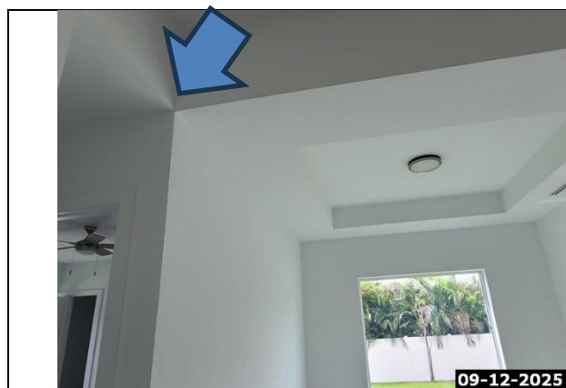
Insufficient Paint at Wall Edges
