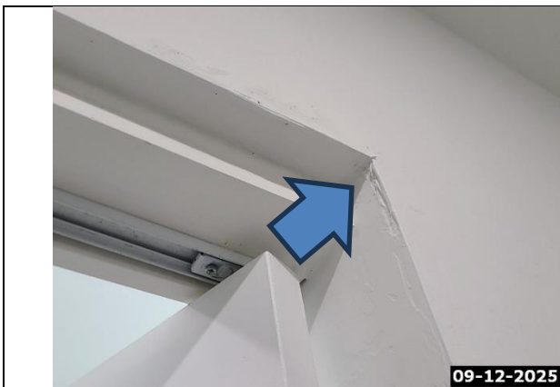
Poor Wall Texture
