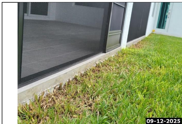
No Stucco at Wall Under Patio
