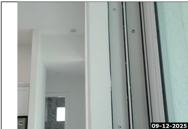
Wall Around Sliding Patio Door Excessive Joint Compound Edges Not Straight
