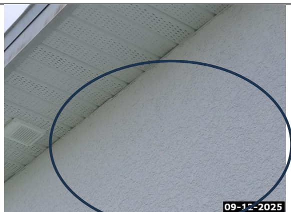
Wall Appears Gray (Not Enough Paint)
