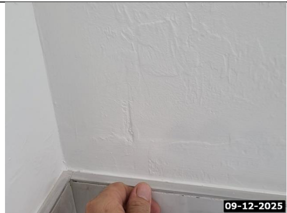
Poorly Installed Wall Texture
