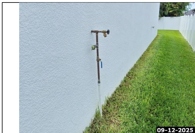
Plumbing – Main Shutoff Valve
