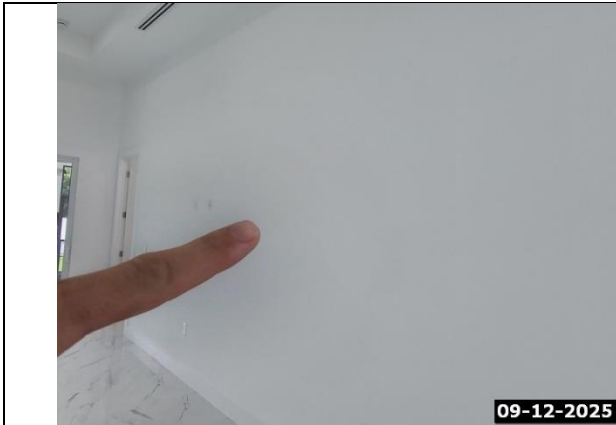
Living Room Wall (North) Gray Areas Visible (Insufficient Paint)
