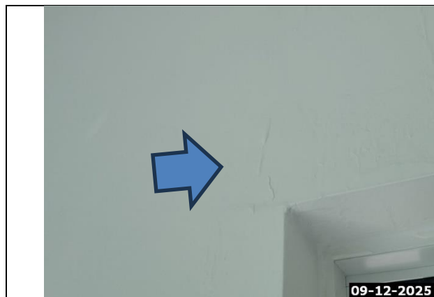
Poorly Installed Wall Texture
