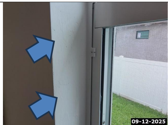
Poorly Installed Wall Texture
