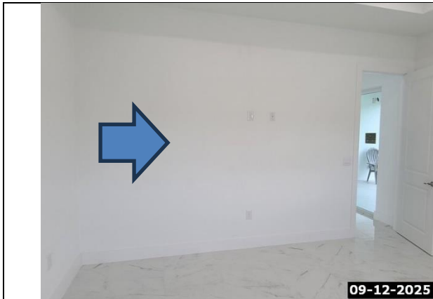
“Gray” Area of Wall (Insufficient Paint)
