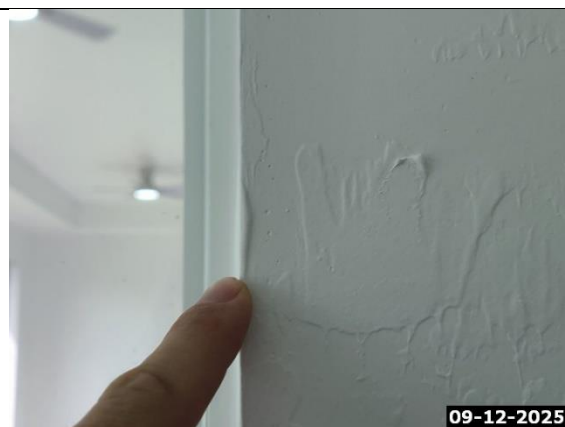
Poorly Installed Wall Texture
