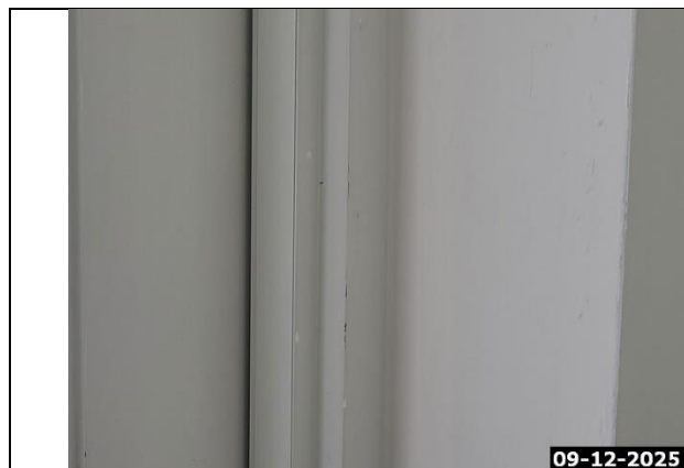
Excess Paint on Different Areas Around Door
