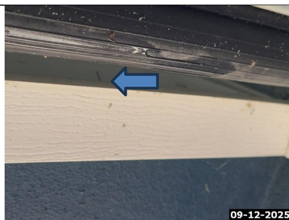
Nails Improperly Installed at Trim Around Garage Door Opening
