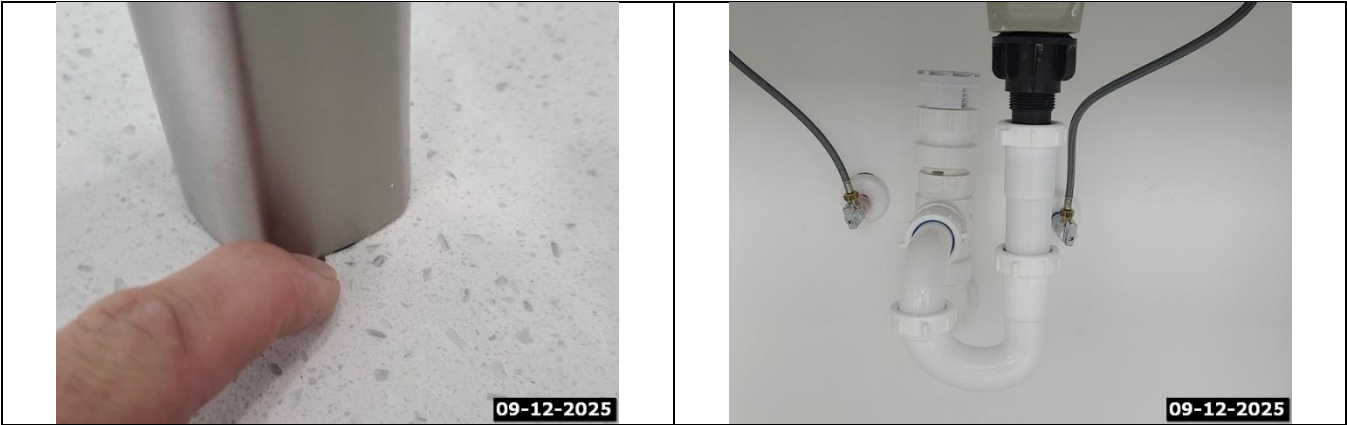
Gap Around Faucet Bathroom #1 Images
