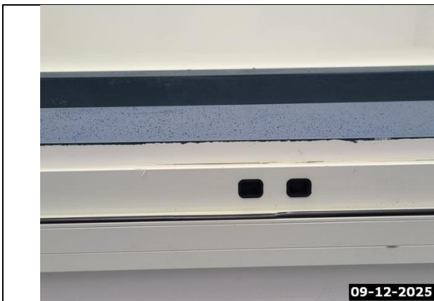
Paint Poorly Installed – Around Door
