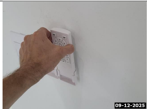
Fan Remotes Tight in Holders
