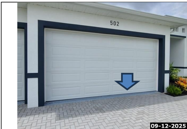
Damaged Slab (Chip)
