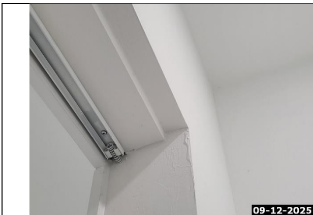
Poorly Installed Wall Texture
