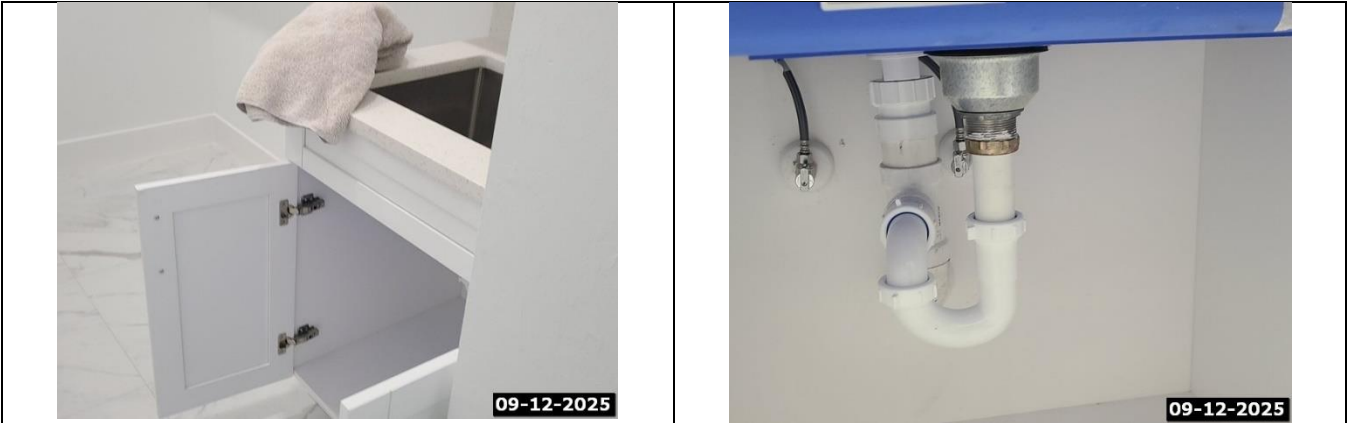
Plumbing System Images Plumbing System Images
