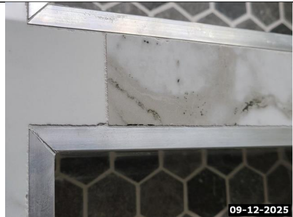
Small Chipping Visible at Edges of Wall Tile at Shower
