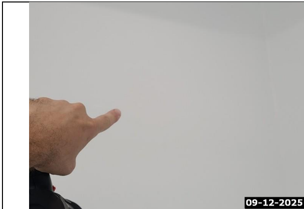
“Gray” Area of Wall (Insufficient Paint) And Poor Wall Texture
