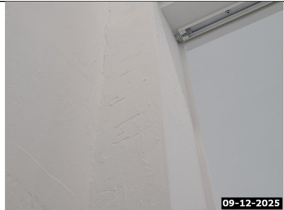
Poorly Installed Wall Texture
