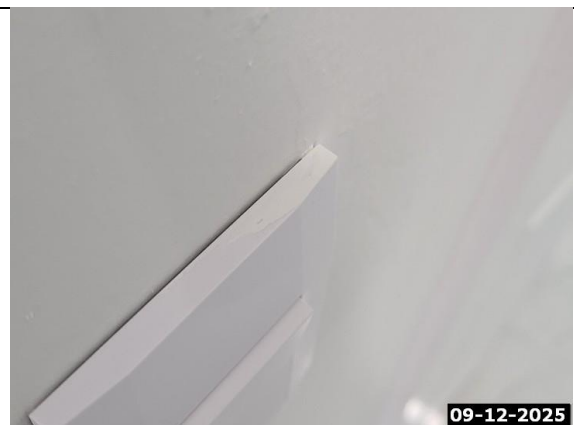
Paint on Hallway Light Switch
