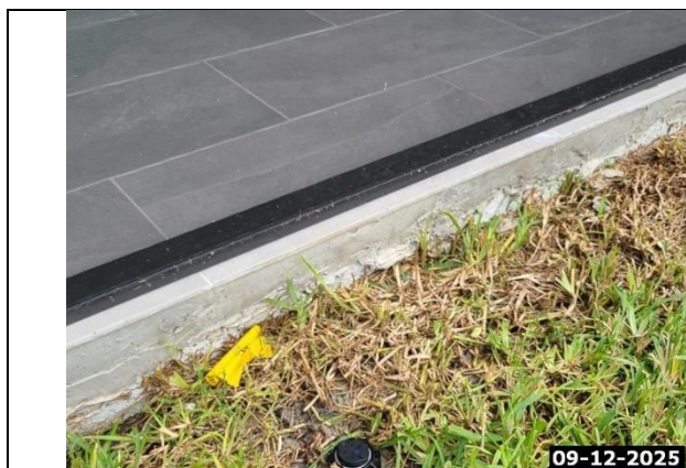
No Stucco at Wall Under Patio
