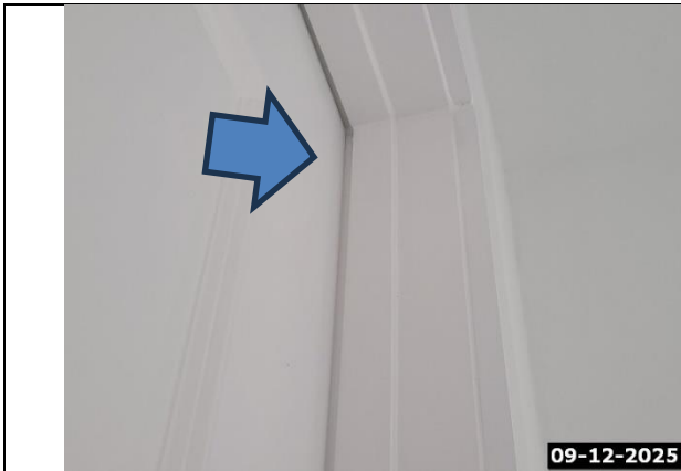
Hall Bathroom Door Appears Warped – Top of Door Bowing Out
