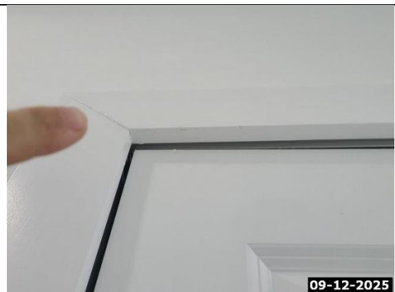
Trim Around Door is Not Aligned
