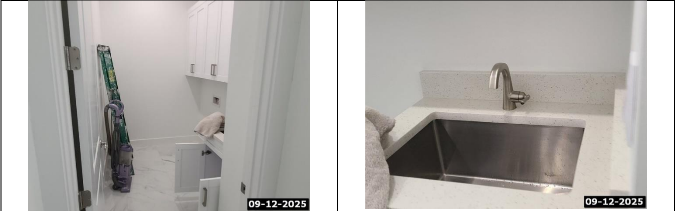
Plumbing System Images Plumbing System Images
