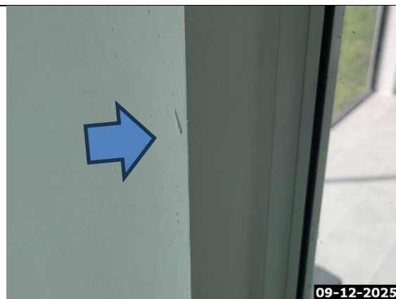
Poorly Installed Wall Texture
