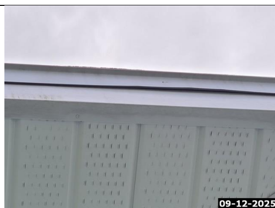
Uneven Gapping at Drip Edge
