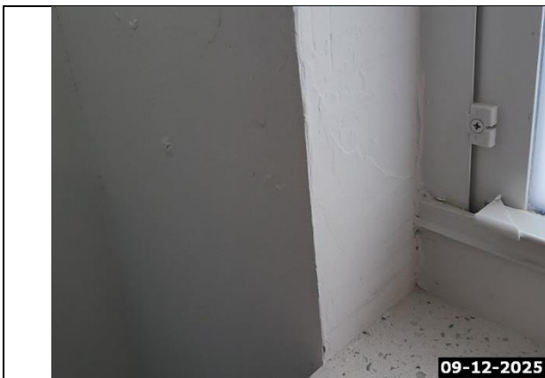
Poor Wall Texture Master Bathroom Window
