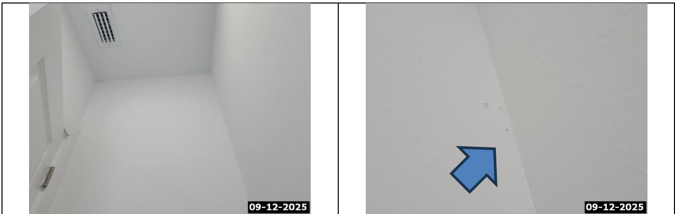
Poorly Installed Wall Texture Master Bathroom Corner Cracking
