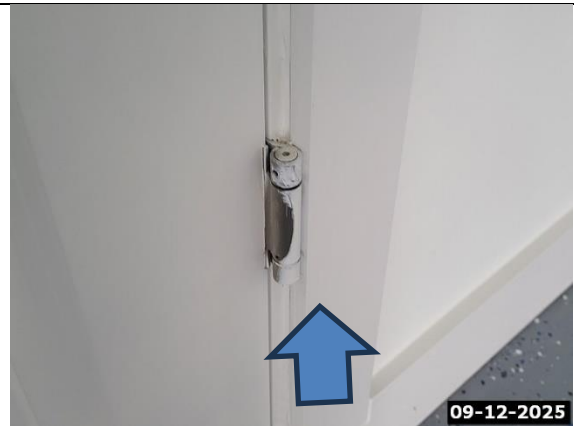
Paint at Hinges
