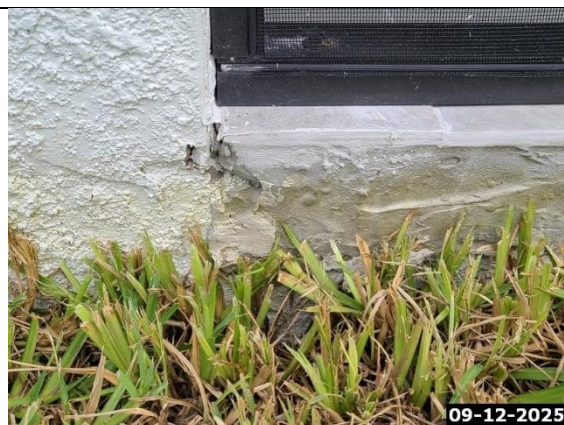
No Stucco at Wall Under Patio
