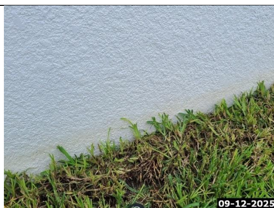
Staining at Bottom of Wall
