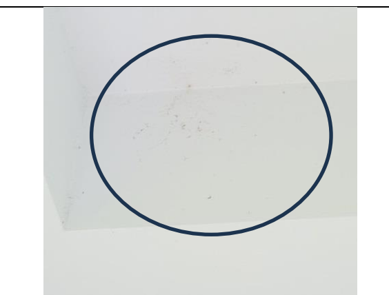
Ceiling – Stains from Insects
