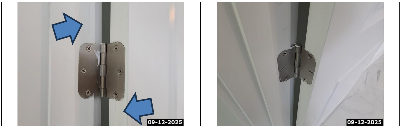
Southwest (left-Rear) Bathroom Cracking at Door Frame and Door
