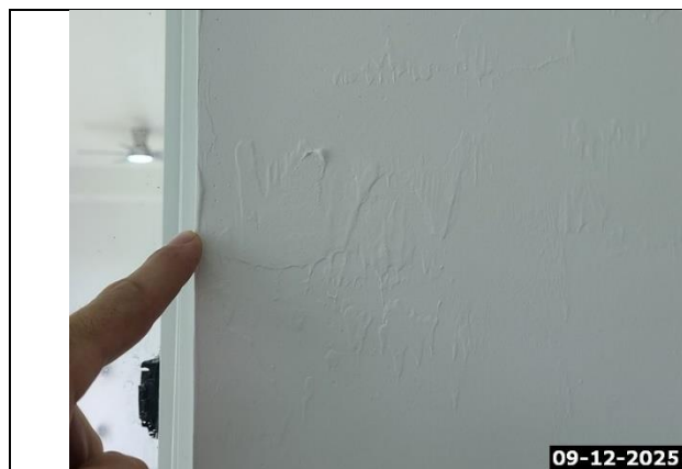
Poorly Installed Wall Texture
