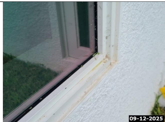
Staining at Seam Under Window Trim
