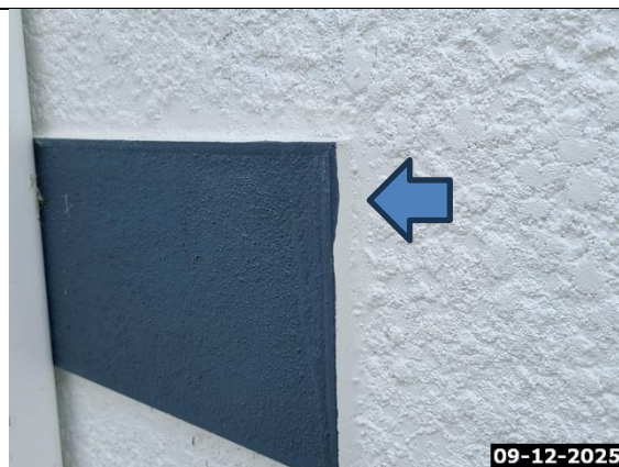
Poor Paint Lines at Transitions
