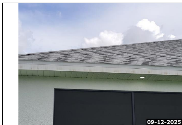
Staining at Fascias
