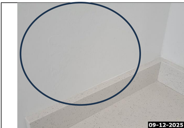
Poorly Installed Wall Texture Left of Master Bathroom Sink
