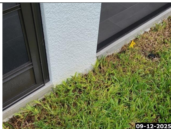
No Stucco at Wall Under Patio
