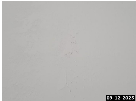
“Gray” Area of Wall (Insufficient Paint) And Poor Wall Texture
