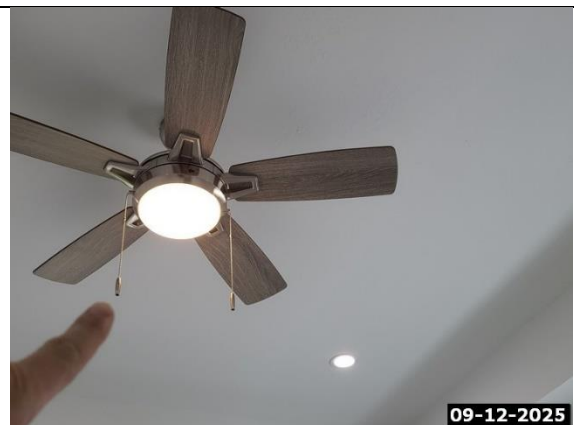
Ceiling Fan Cords Too High
