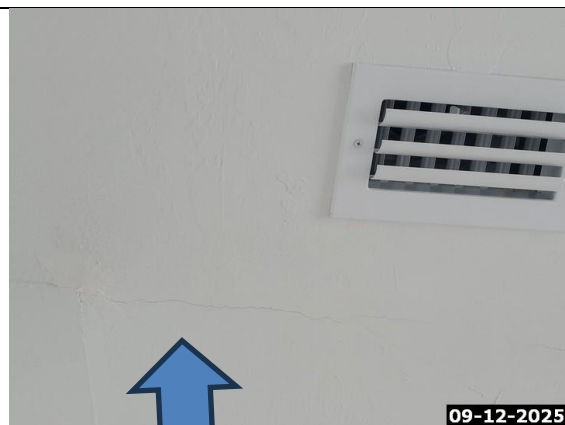
Cracking at Ceiling Master Bathroom
