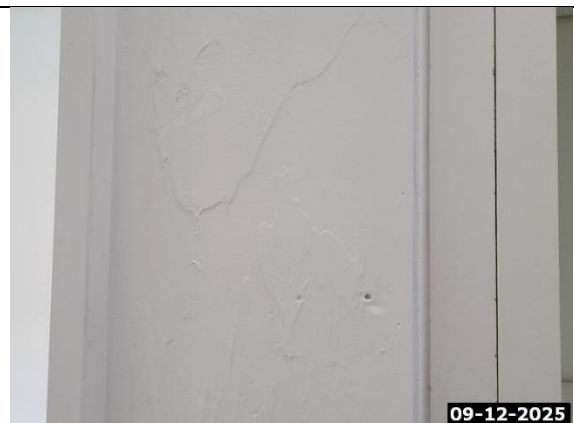
Poorly Installed Wall Texture
