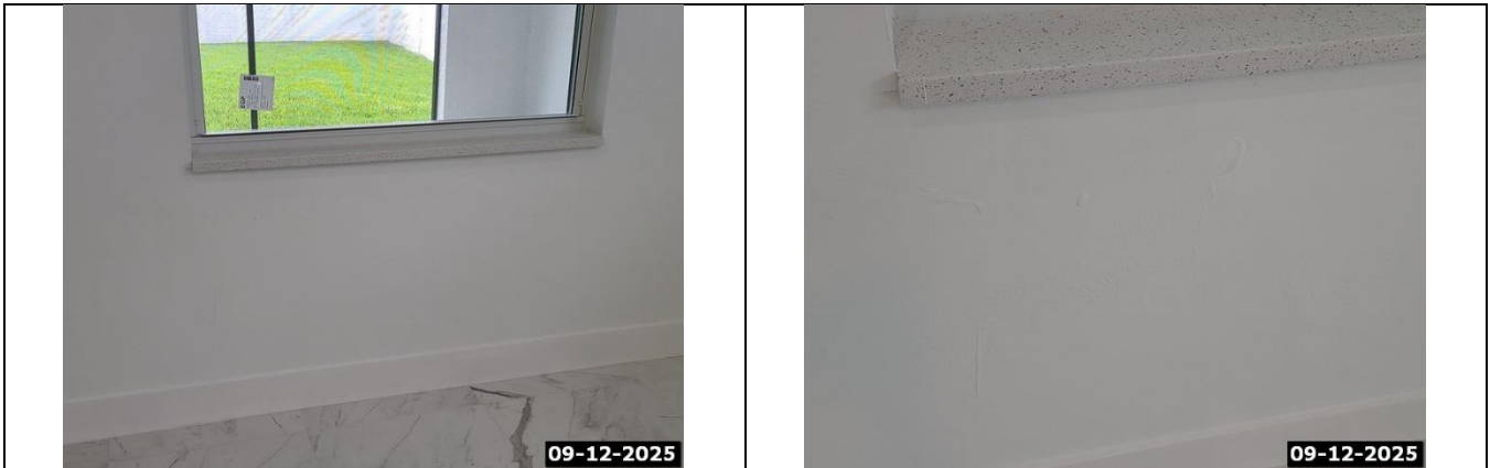
Poor Wall Texturing
