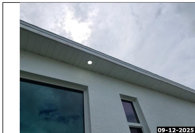
Staining at Fascias
