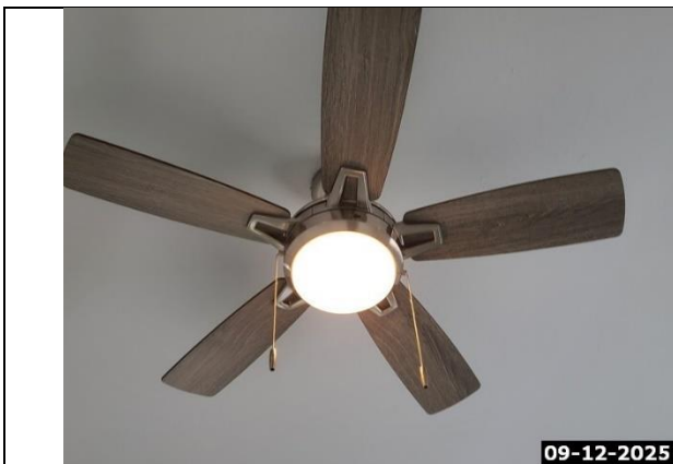
Ceiling Fan Cords Too High
