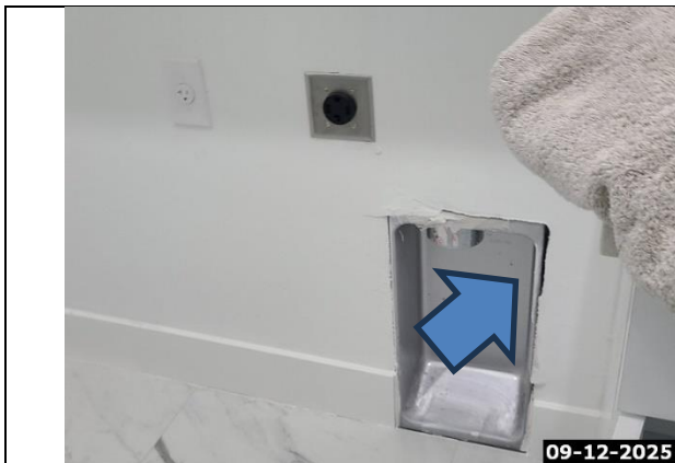
Poorly Installed Wall Texture
