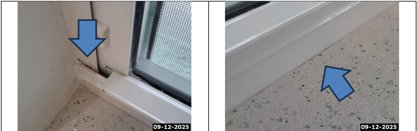
Caulking separated at Window Frame
