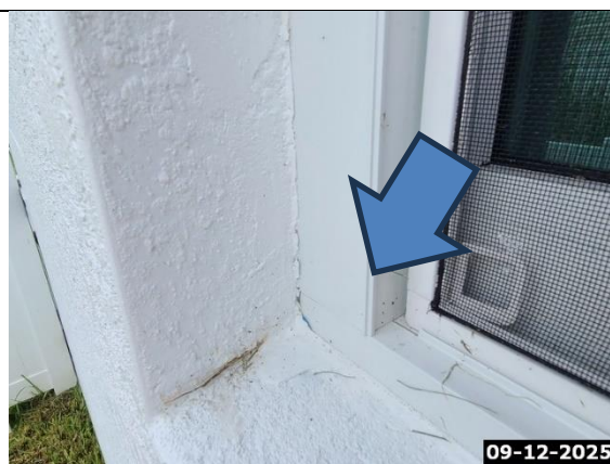
Cracking at Window Sealant
