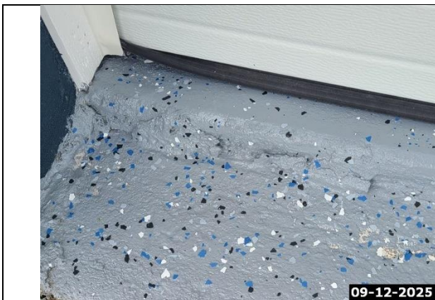
Debris Under Coating (Uneven)
