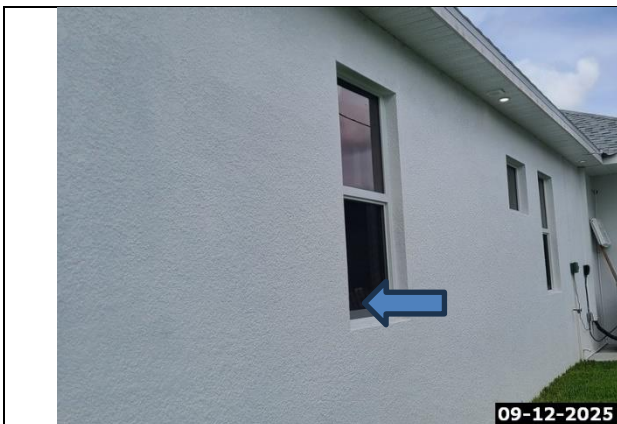
Cracking at Caulking
