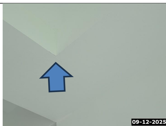
Insufficient Paint at Wall Edges
