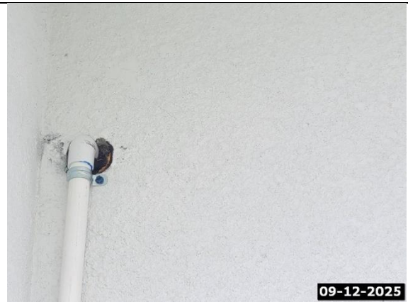
Gaps Present around AC System Condensation Drain Line
