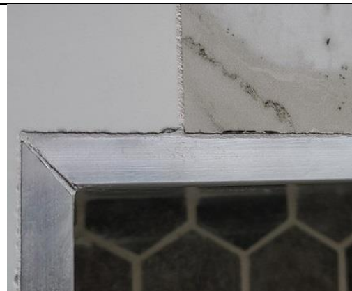
Small Chipping Visible at Edges of Wall Tile at Shower
