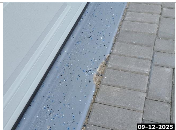
Damaged Slab (Chip)
