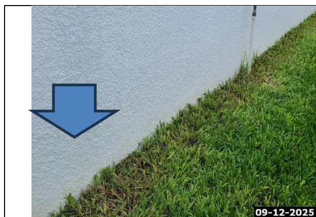
Staining at Bottom of Wall
