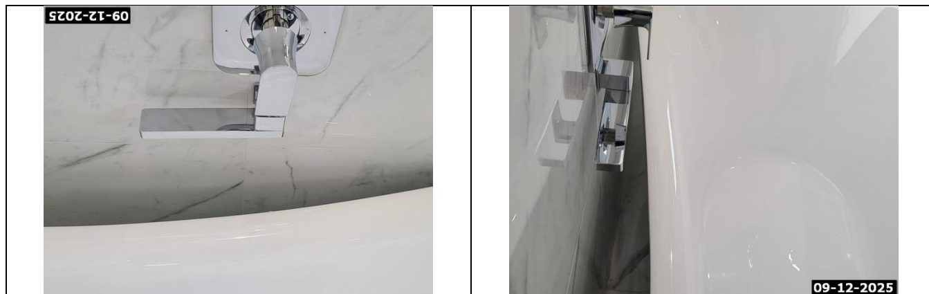
Bathtub Faucet – Faucet Turns Enough to be Outside of Bathtub
