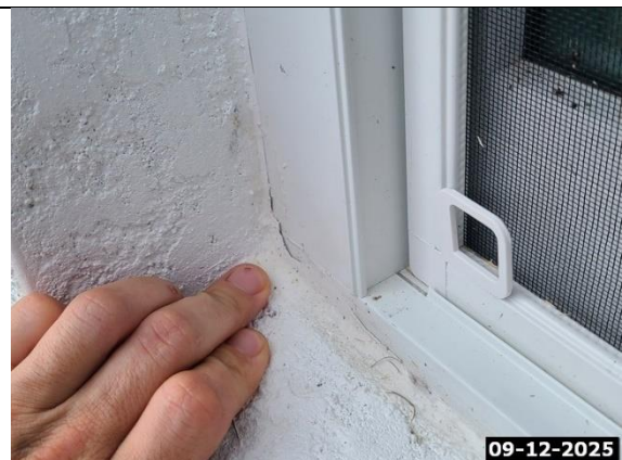
Cracking at Caulking
