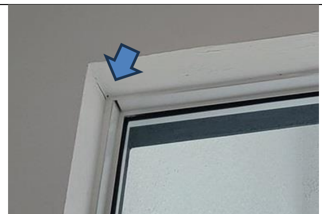
Cracking at Wall Around Window
