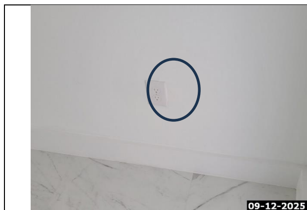
Wall Repair Visible Around Outlet Next to Front Entry
