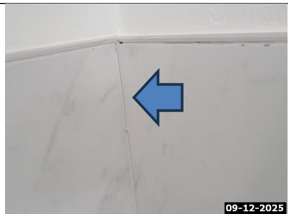
Cracking at Grout / Caulk at Corner Seam of Wall Tile
