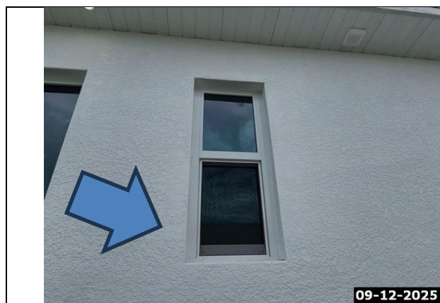
Cracking at Window Sealant
