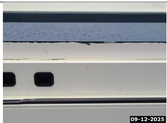
Paint Poorly Installed – Around Door
