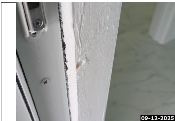
Wall Around Sliding Patio Door Excessive Joint Compound Damage Present
