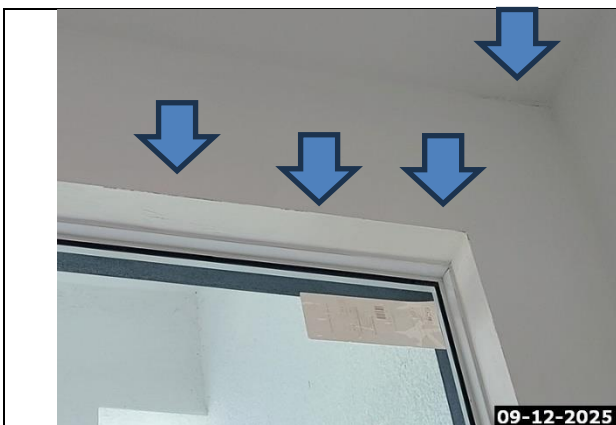
Exposed Corner Bead at Window + Lack of Paint at Wall Corner
