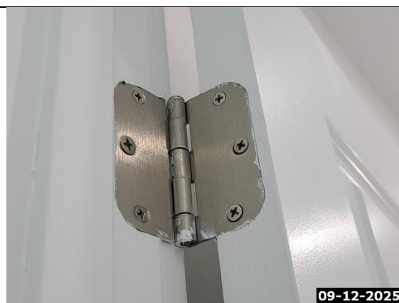
Paint at Door Hinges
