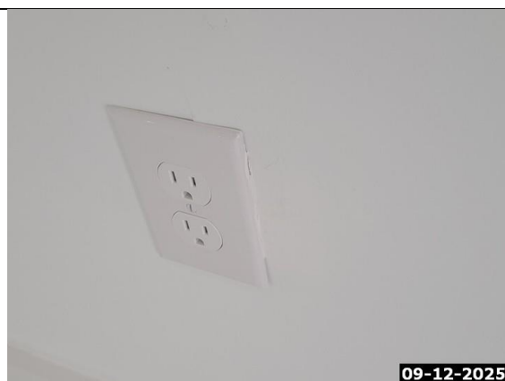
Wall Repair Visible Around Outlet Next to Front Entry
