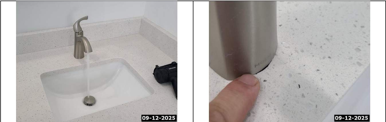
Bathroom #1 Images Gap Around Faucet
