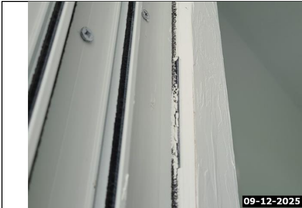
Wall Around Sliding Patio Door Excessive Joint Compound Joint Compound Falling Away
