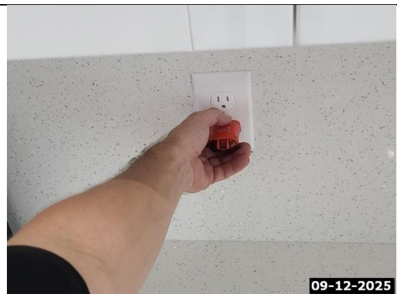
GFCI Protection at Electric Panel
