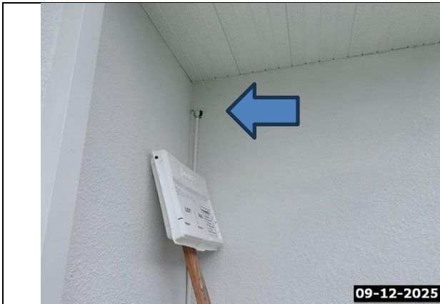
Gaps Present around AC System Condensation Drain Line
