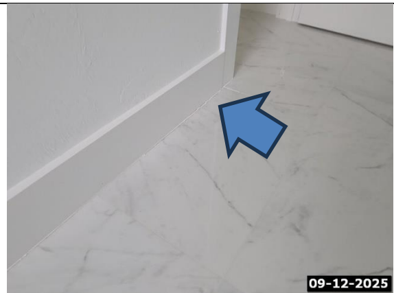
Caulking Cracking Between Wall Moulding and Floor Tile
