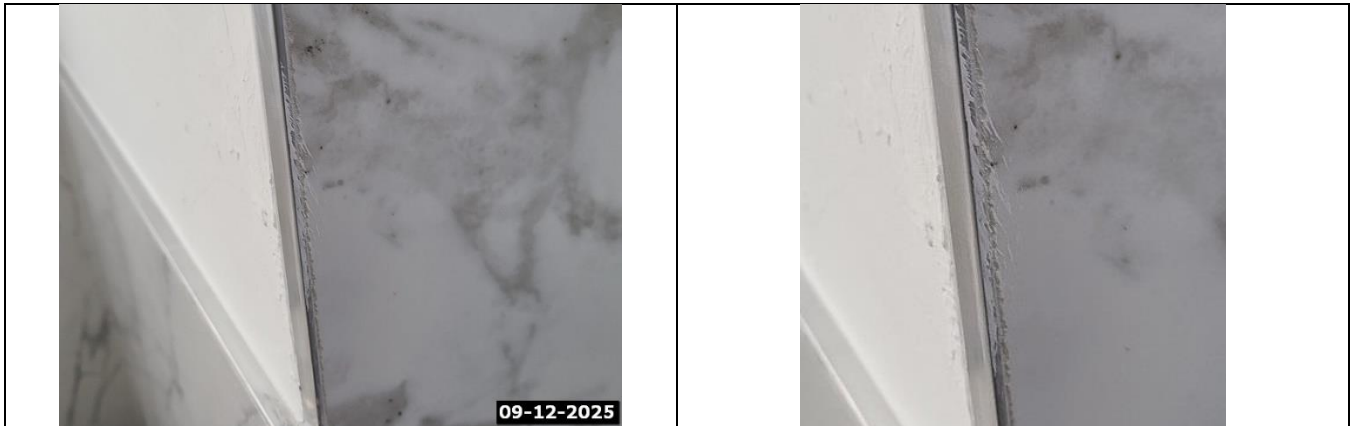
Paint / Debris on Shower Tile
