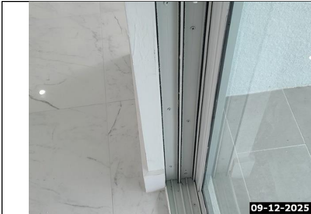
Wall Around Sliding Patio Door Excessive Joint Compound Edges Not Straight
