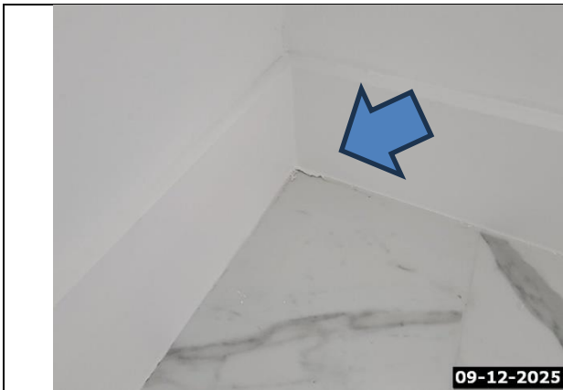
Caulking Cracking Between Wall Moulding and Floor Tile
