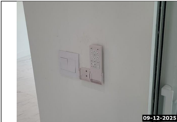
Fan Remote Holders Not Properly Installed
