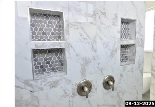
Tiles Edges Rough Where Cuts Were Made
