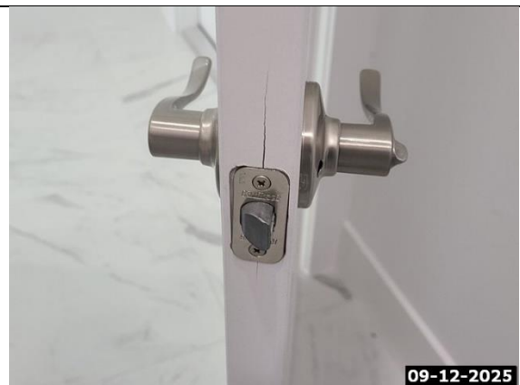
Cracked Door at Latch Bore Laundry Room
