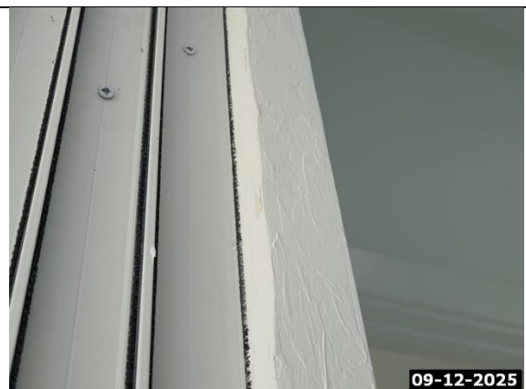
Wall Around Sliding Patio Door Excessive Joint Compound Edges Not Straight
