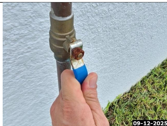
Plumbing – Main Shutoff Valve Rust at Nut Securing Handle
