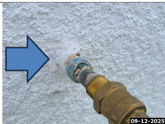
Cracking at Sealant
