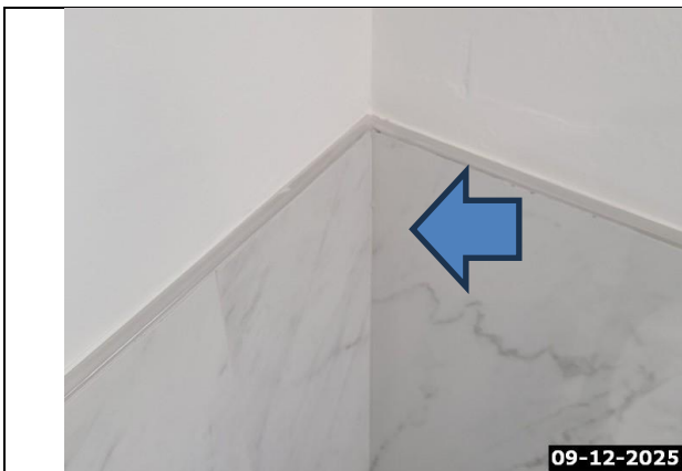
Cracking at Grout / Caulk at Corner Seam of Wall Tile
