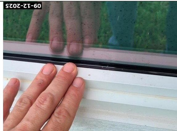
Rear Fixed Window – Standing Water at Bottom Seal
