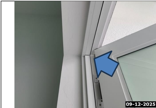
Gap at Door Frame
