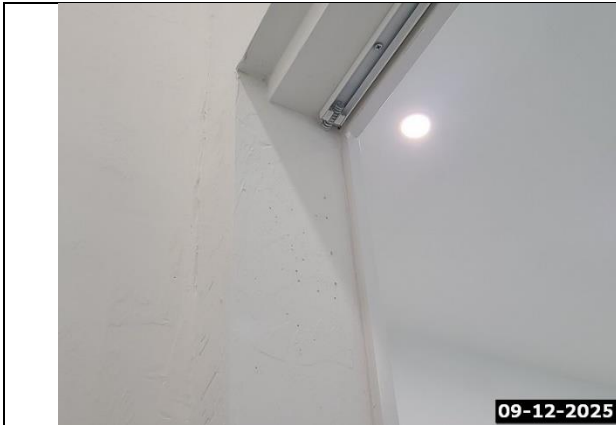
Poorly Installed Wall Texture
