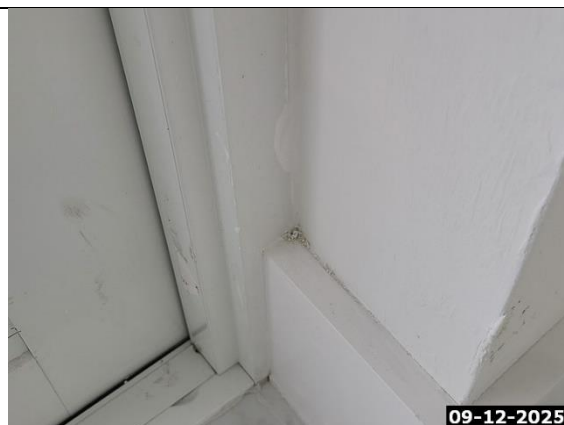
Excess Paint on Different Areas Around Door
