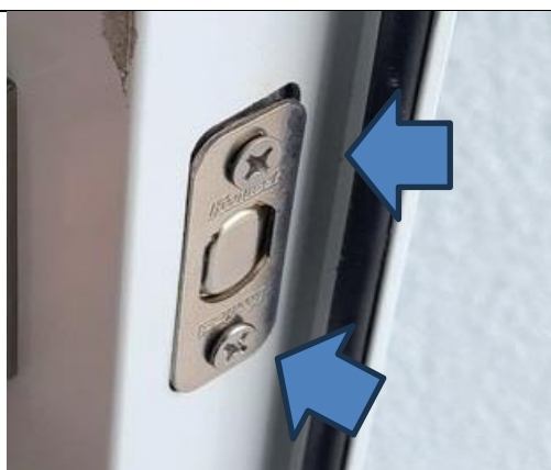
Strikeplate and Hardware Not Flush
