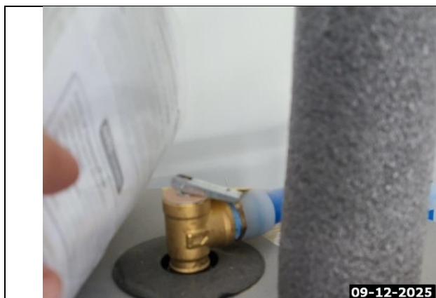
Water Heater Relief Valve (TPRV)
