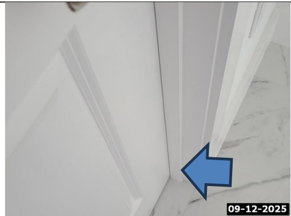
Hall Bathroom Door Appears Warped – Bottom of Door in Contact with Frame
