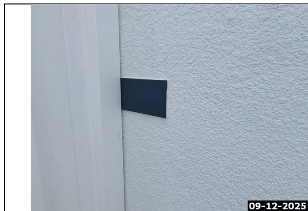
Poor Paint Lines at Transitions
