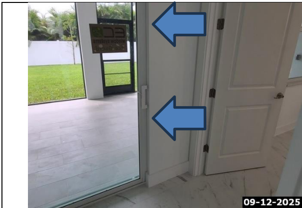
Wall Corner Falling Apart Near Sliding Patio Door
